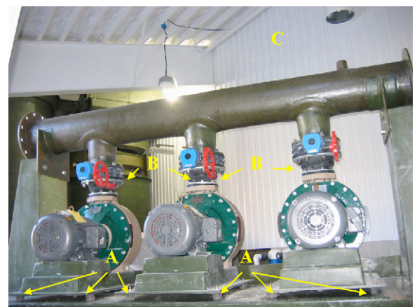
Fig. 8. A custom pump stand fabricated by Marine Biotech Inc. (Beverly, MA) installed at the USDA ARS, NCSWAC (Franklin, ME) illustrates (A) resilient pump mounts to reduce transmission of motor vibration noise, (B) rubber vibration isolation couplings on both the pump inlet & outlet piping, and (C) locating the water treatment pumps and equipment in a room separate from the fish culture tanks.
